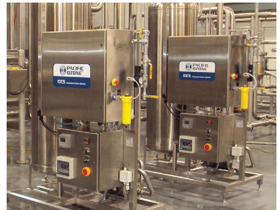
NSGA shown on complete system retrofit for bottle water application
